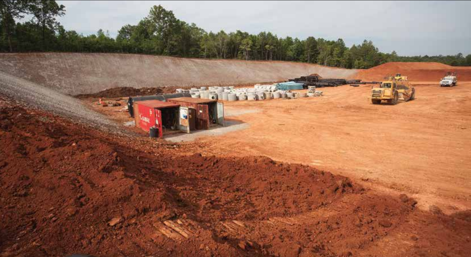
The site had to be cut to a 30-foot-plus depth in some places.
